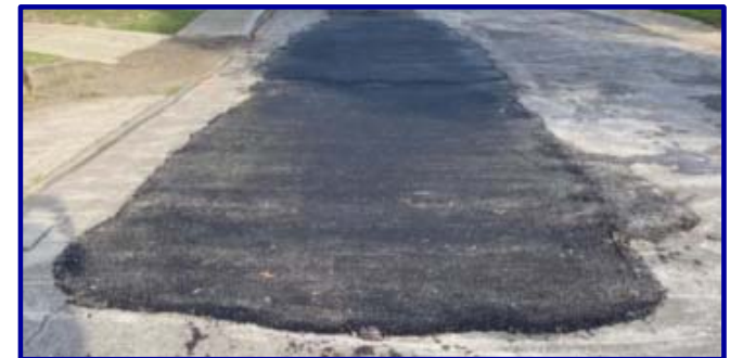
Pavement Patches on Senisa Drive
